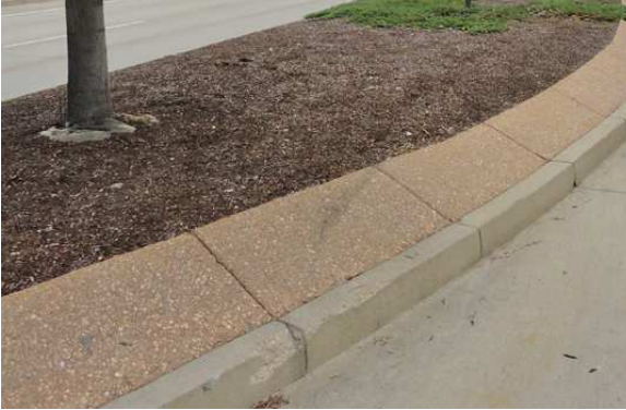
Sloped splash block design: existing Standard Arterial Streetscape corridors throughout the city include extensive segments with existing sloped concrete splash blocks, per a former standard.
