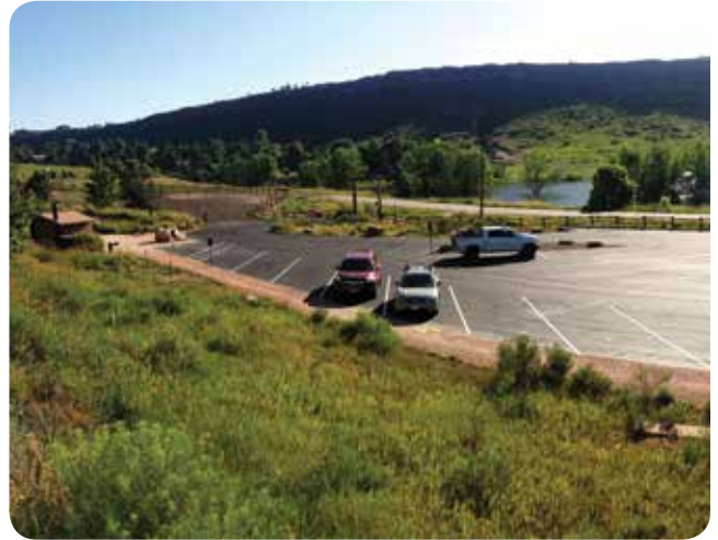
Larimer County crews completed most of the work on the remodeled Soderberg Trailhead, saving taxpayers thousands of dollars. Photo © Steve McCorkel
